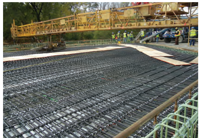
Placing carbon-fiber-composite cable reinforcements in the deck of the M 102 bridges over Plum Creek in Michigan.
