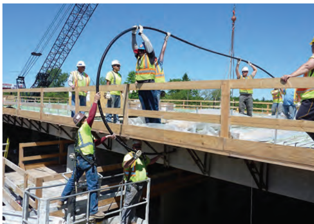
Passing carbon-fiber-composite cable strand through conduit for the Interstate 94 bridges over Lapeer Road in Michigan.
