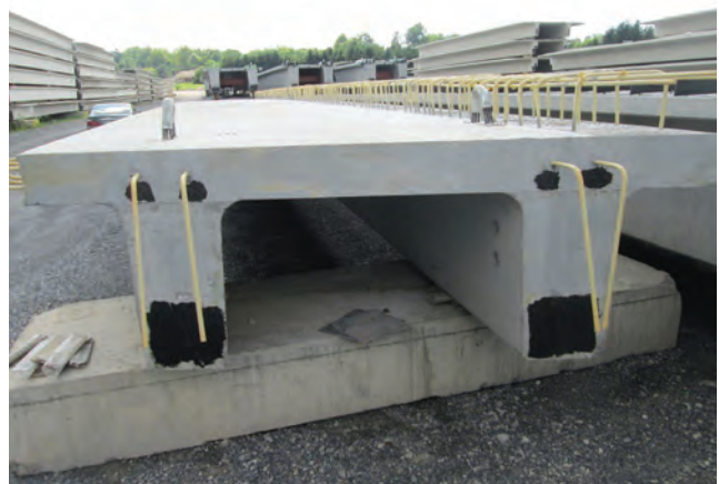
Completion of northeast extreme tee beam for the Kittery overpass bridge in Maine.
