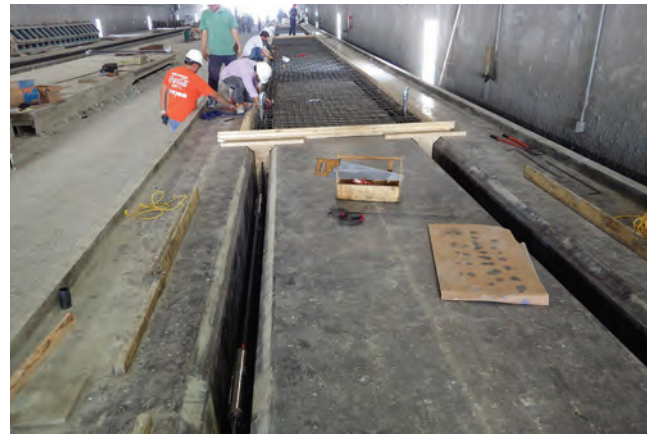
Carbon-fiber-composite cable strands in the stem for the Innovation Bridge in Florida.
