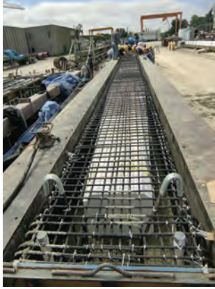
Prestressing bed with carbon-fiber-composite cable from the M102 bridges over Plum Creek in Michigan.
