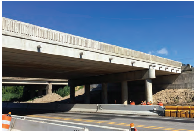
Completion of the eastbound Interstate 94 bridge over Lapeer Road in Port Huron, Mich.
