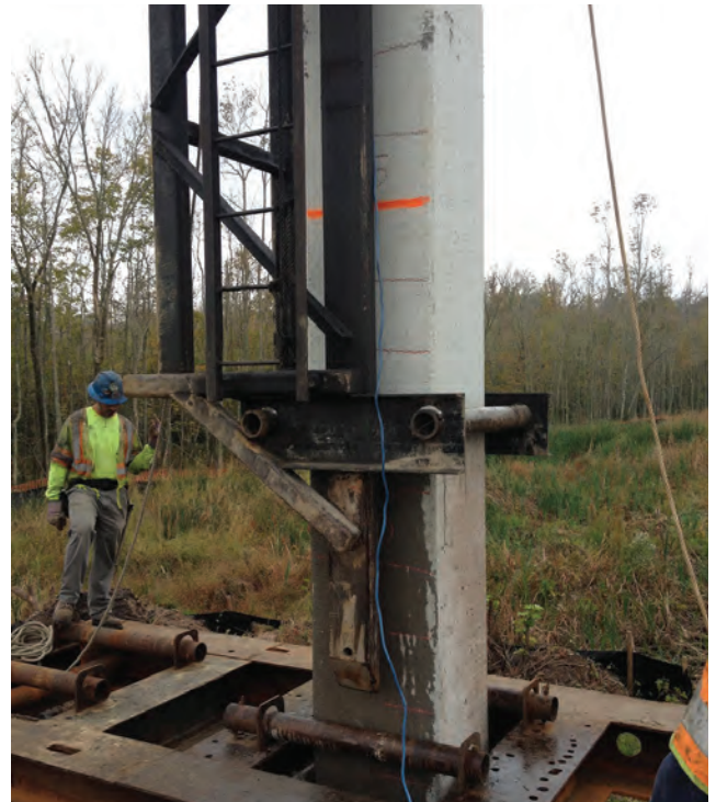
Driving test of the precast concrete pile for the Nimmo Parkway bridge in Virginia.
